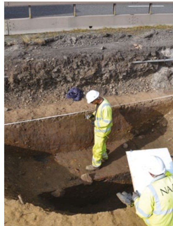
Excavations taking place on one of the large Roman watering holes at the Scurragh House site.
